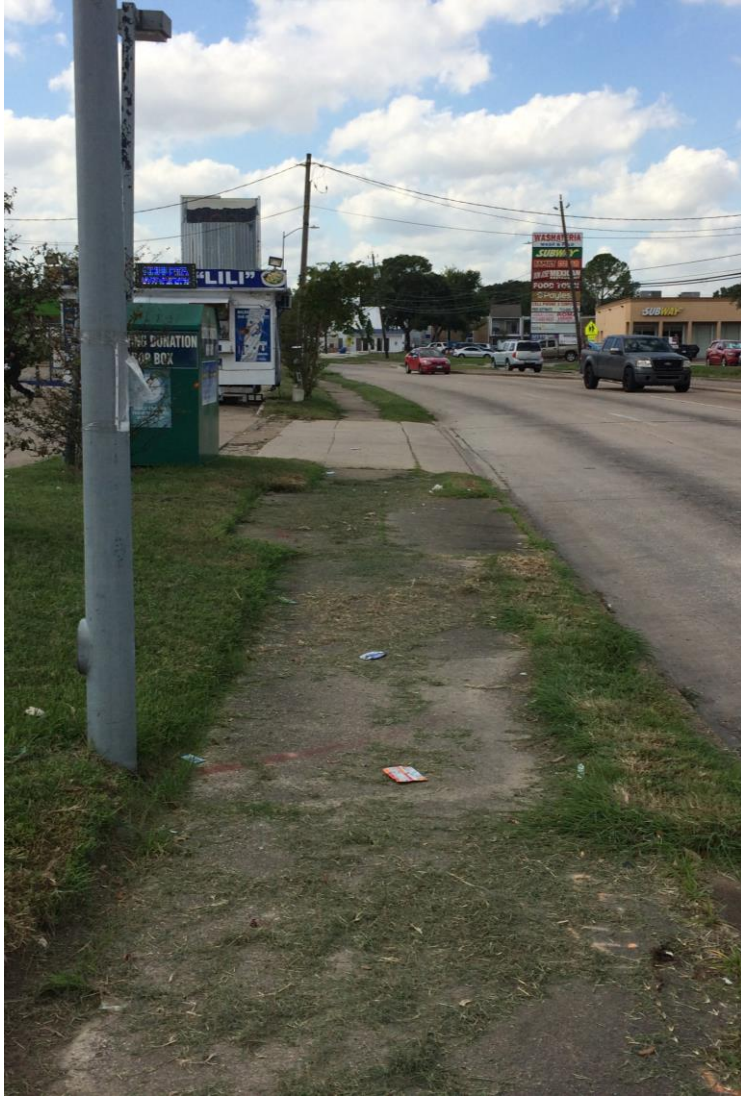
Sidewalks - Poor Condition
