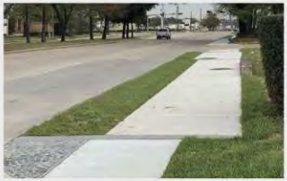
Sidewalk with planting strip completed on W Little York near Langfield Rd
